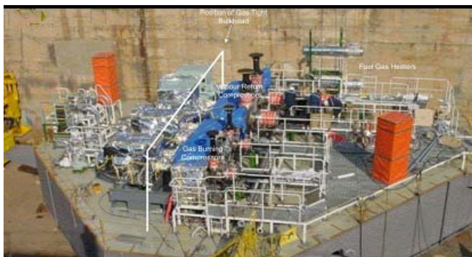
Figure 4.2: Typical compressor room
